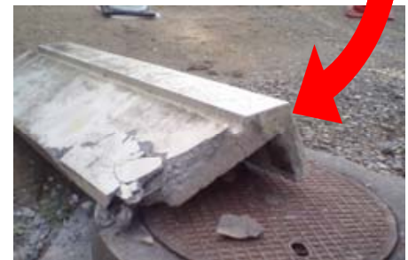
A railing has fallen due to deterioration
