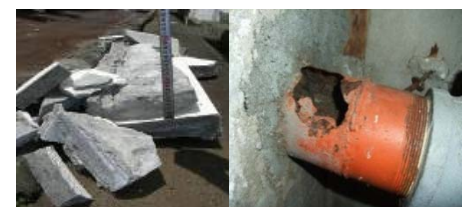
(Left) Fallen mortar (Right) Damage to pipework due to degradation
