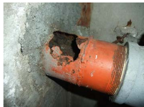
Damage to pipework due to degradation
