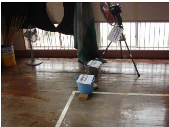
Damage to the ceiling and floor boards due to a rainwater leak (29-year-old building)
