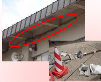
Fallen concrete slabs due to deterioration
