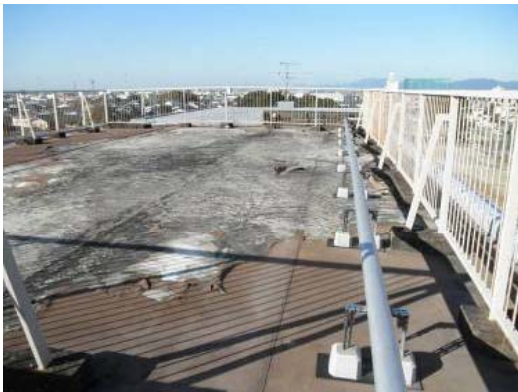
Deterioration of the waterproof layer. Water leaked inside, damaging the ceiling and floor of a corridor (37-year-old building)
