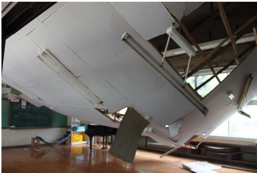
Corroded wooden hanging material fell from the ceiling due to a rainwater leak (50-year-old building)
