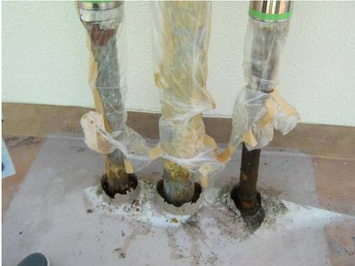
Corrosion of steel pipes for fire extinguishing due to erosion by rainwater (38-year-old building)
