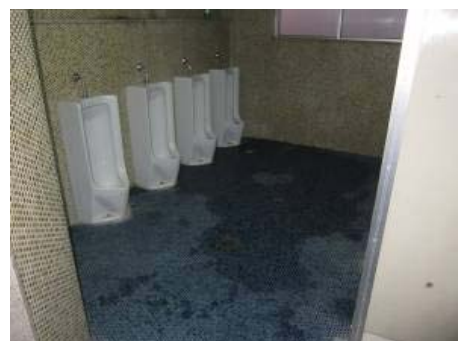
A bad smell due to the deteriorating toilet
