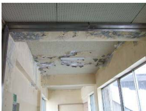
Deterioration of the ceiling due to a rainwater leak (38-year-old building)
