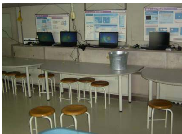
Broken computers due to a rainwater leak
