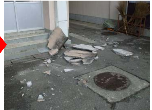
Fallen mortar slabs (31-year-old building)
