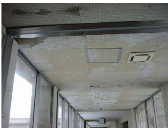
Deterioration of the ceiling due to a rainwater leak (31-year-old building)
