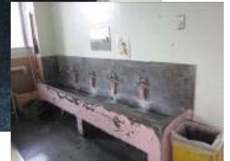
Toilet odor due to deterioration
