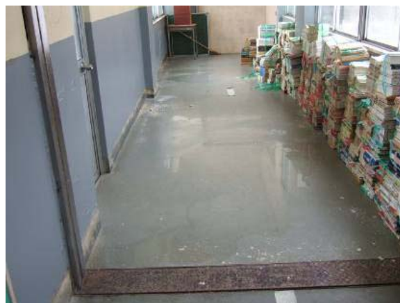
Rain-soaked floor (38-year-old building)
