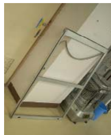
Fallen window frame
