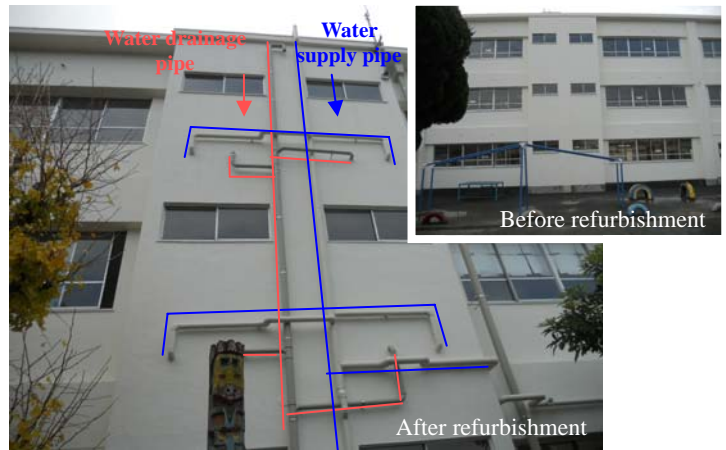
Pipework exposed during the refurbishment of pipework for the sink at the corridor
