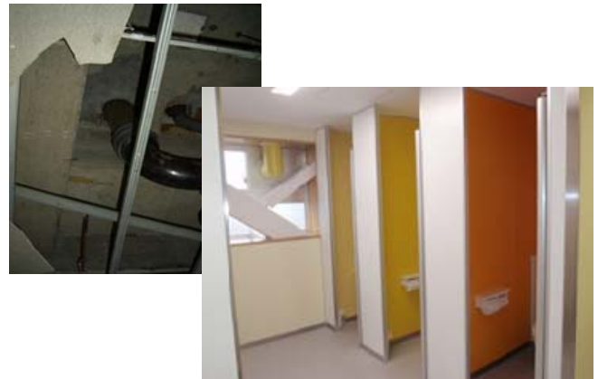
Figure 2: Left: Leaking toilet pipework; Right: Toilet after maintenance and repair
