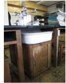
Pipes break quite often
