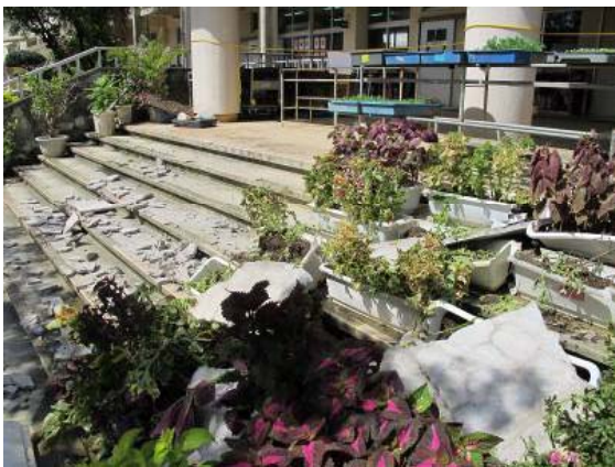
External mortar peeled off and lightly injured a student (29-year-old building)
