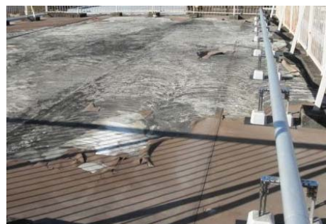
Frequent leaking caused by the degradation of the waterproof finish due to deterioration
